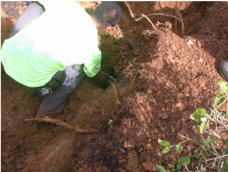
Rotten Concrete Pipe
