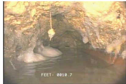
Grease on the walls of a sewer pipe
