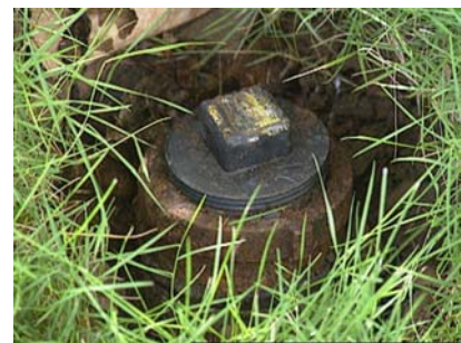
Typical sewer cleanout with properly installed plug.
