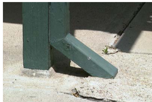
Example of downspout potentially connected to the sewer.
