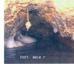
Grease on the walls of a sewer
