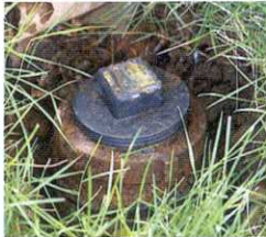
Sewer cleanout with properly installed plug
